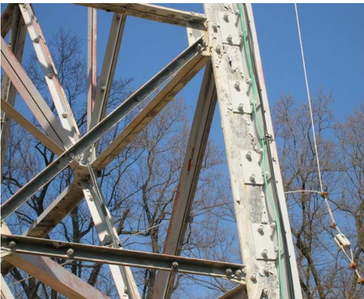
Peeling lead paint is visible on this section of the tower.
